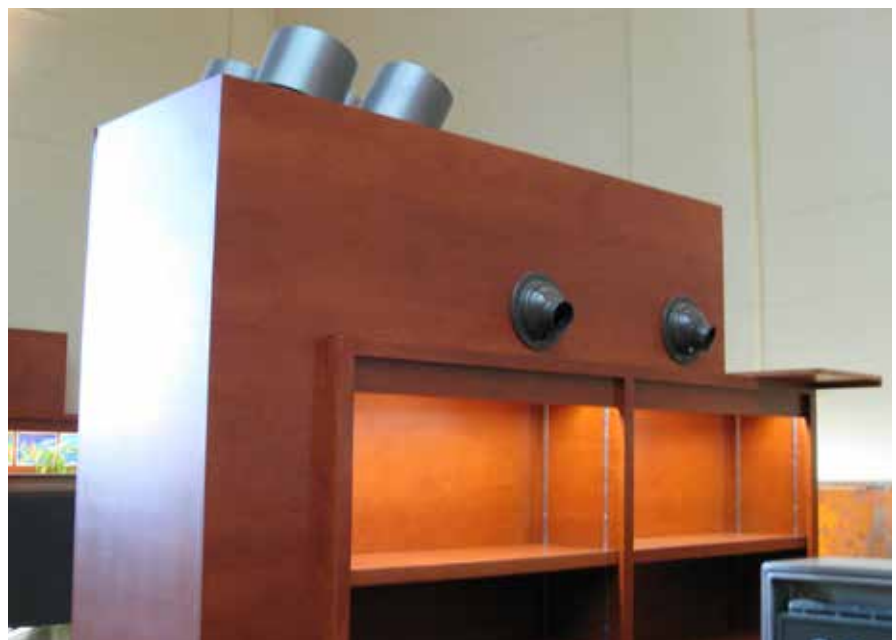
Directional localized Punkah grilles integrated into modern furniture insertions within a voluminous former banking hall. Library of Parliament Annex (Former Bank of Nova Scotia Rehabilitation), Ottawa, ON. MTBA Inc.
