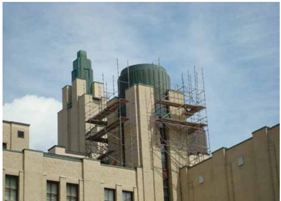
On-going rehabilitation on the exterior masonry wall envelope. Universite du Montreal. Montreal, QC. MTBA Inc.
