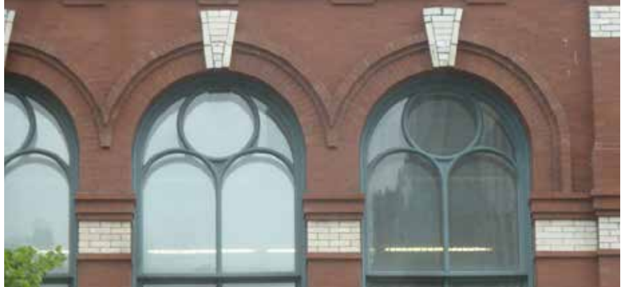
King St. window detail. Energy panels were installed on the interior to improve thermal performance while also retaining these character-defining elements. Jim Bezanson.
