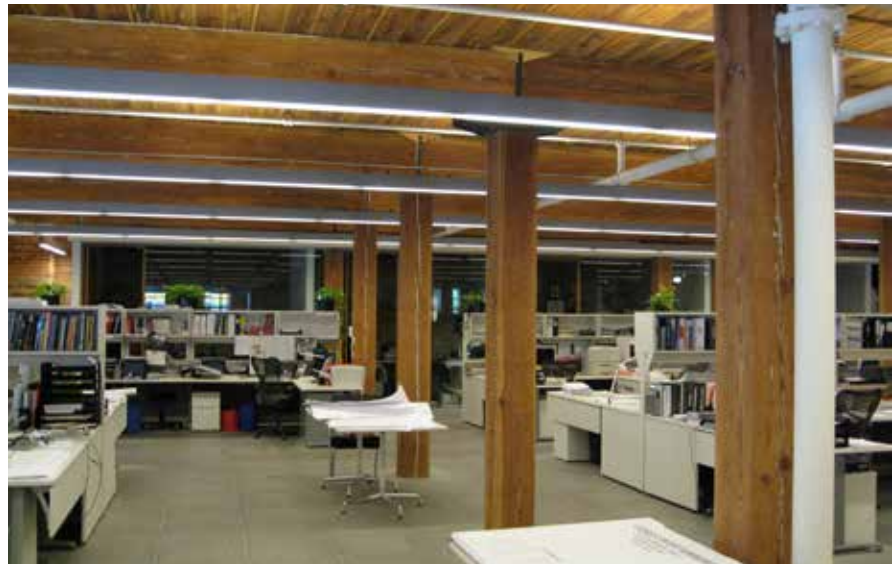
The wood structure and flooring system were retained in adaptive reuse. Former McGregor Sock Factory (Stantec Offices) Toronto, ON. MTBA Inc.
